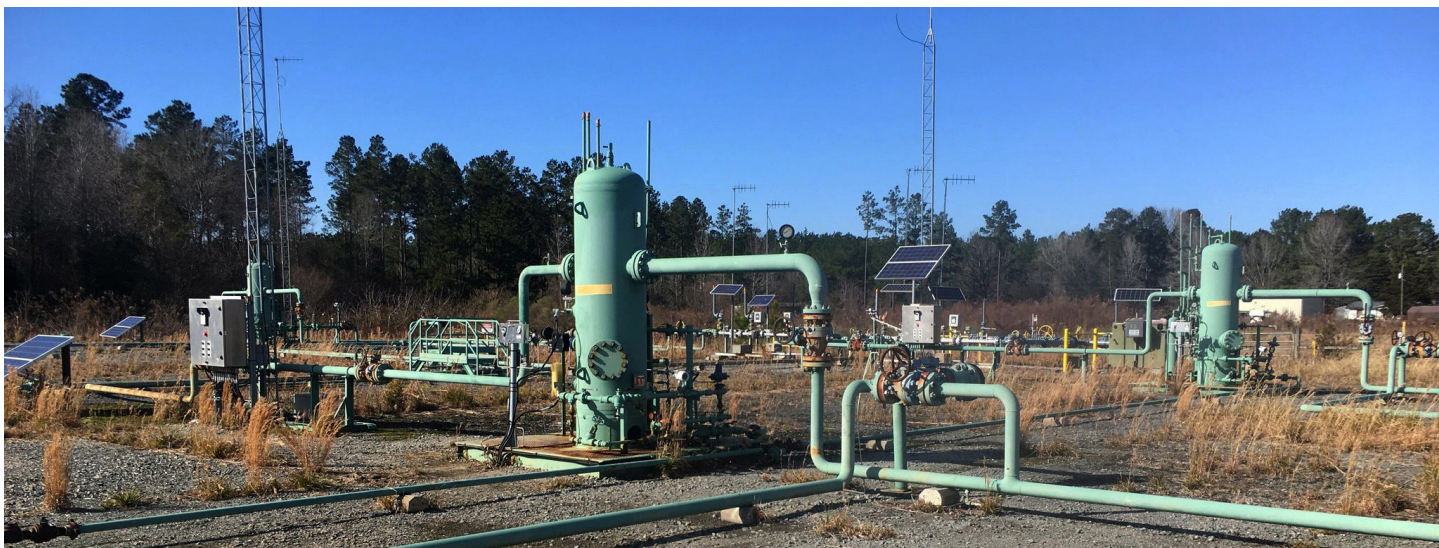
AgoraGateways automate and optimize the choke setpoint on gas wells in the Haynesville Shale.
